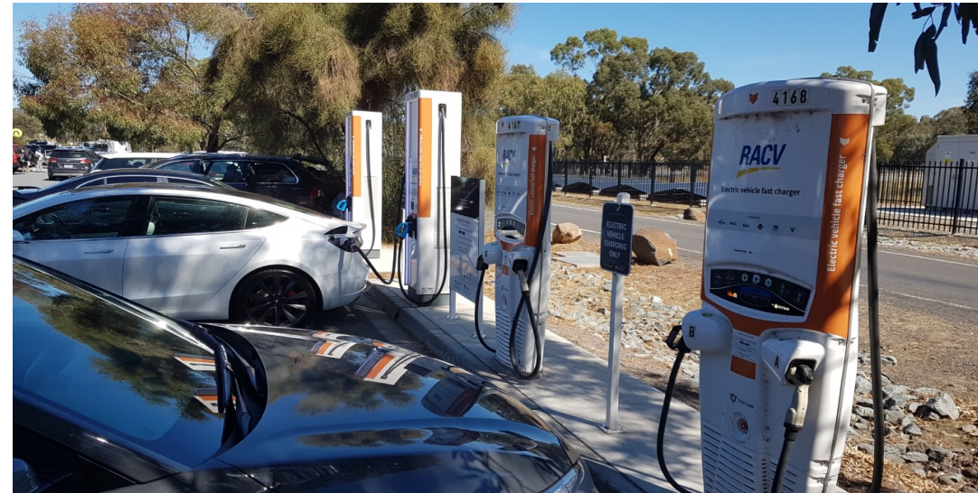
Chargefox Euroa DC 50kW chargers on the right. DC 350kW chargers on the left. All have a choice of CCS Type 2 or CHAdeMO tethered leads.
